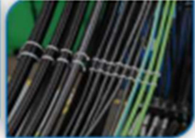
Neat pipe layout
